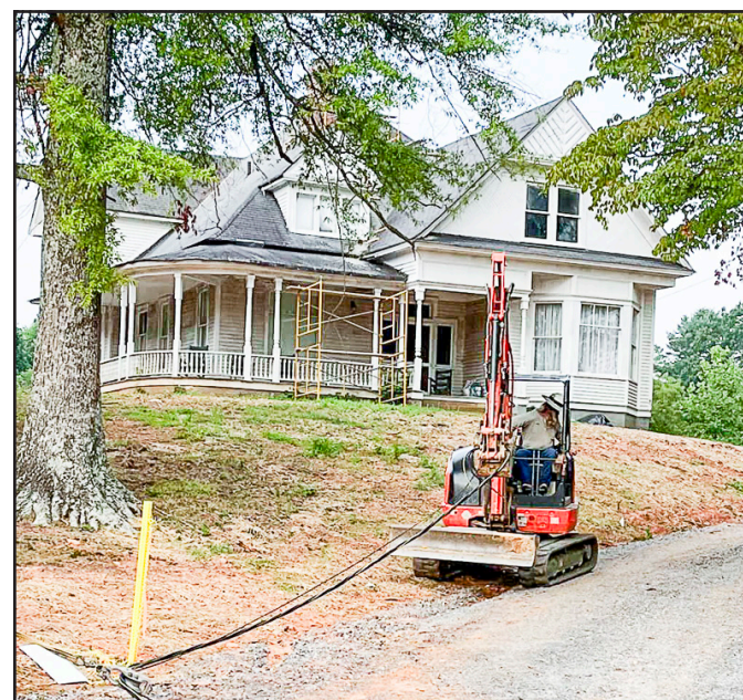
A Blue Ridge Mountain EMC crew running line for the new underground power and fiber cables at the Berrong-Oakley House.
